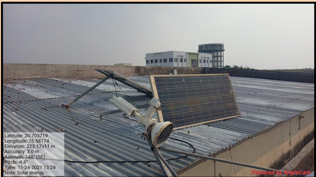
Solar Panel kept on college Building Terrace
